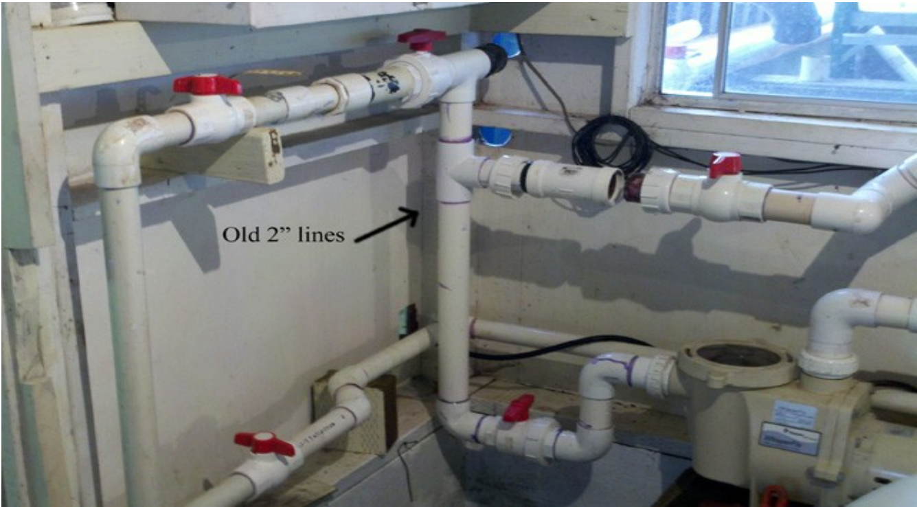
These are the old 2" lines feeding the two filters. The flow is being restricted by the small lines coming from our two water supplies to the east of the hatchery building.
